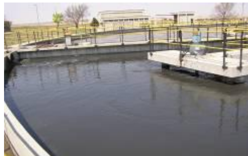
F. New stirrer installed once the effluent was thin enough
