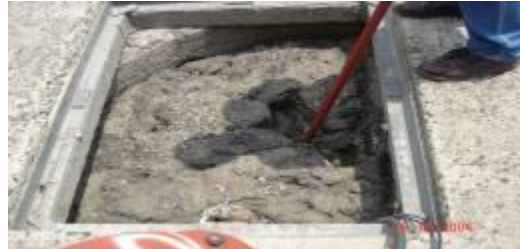
E. Congested pump well that caused the problem. Dosing was implemented
