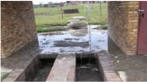
B. The congested well and flow to pump
