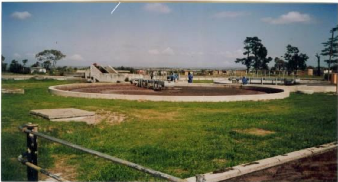
Congested primary clarifier
